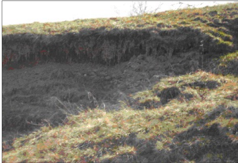
Figure 7. Landslides – Boțești village.
