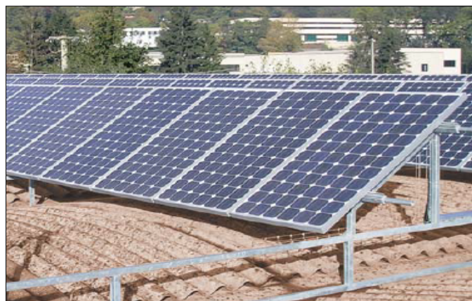
Figure 2. Photovoltaic solar panels.
